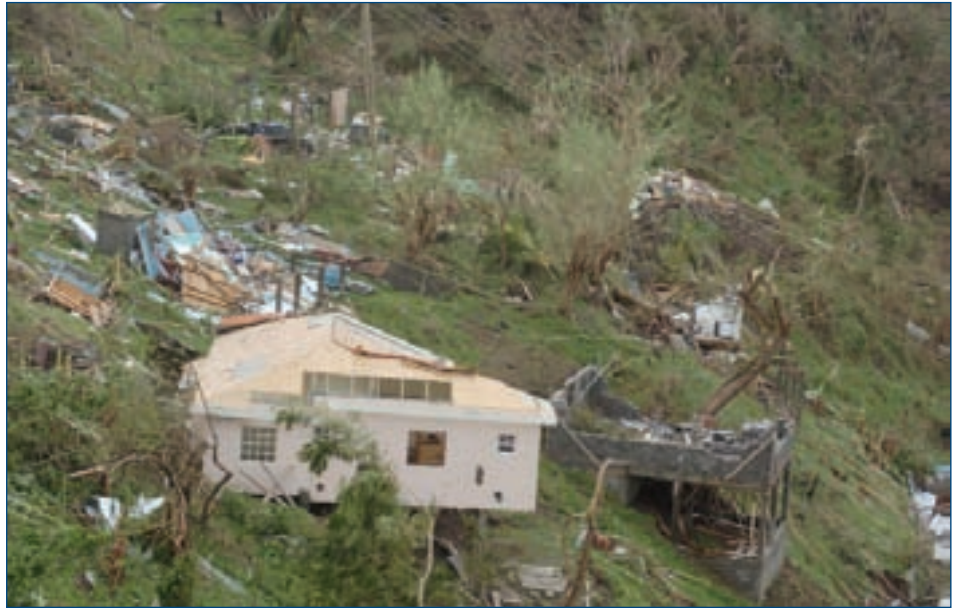
Hurricane damage in Grenada in 2004: more than 90 per cent of the island's buildings were destroyed.
